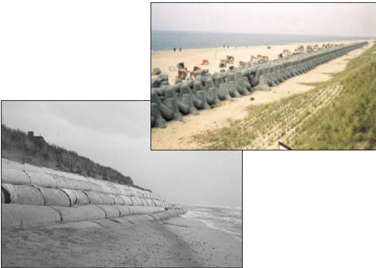
Fig. 8: Examples of hard measures at the western coast of Sylt: tetrapod dune foot revetment at Hörnum and geotextile revetment at Kliffende, Kampen.
